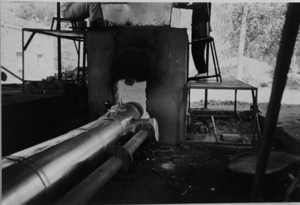
Gasifier-powered Syrup-making Furnace
